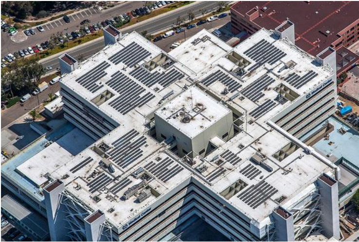
USVA Rooftop Solar
