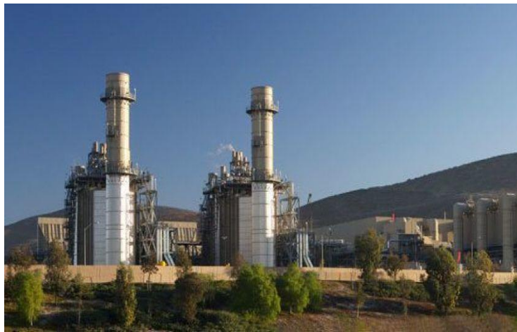
Otay Mesa Generating Project
